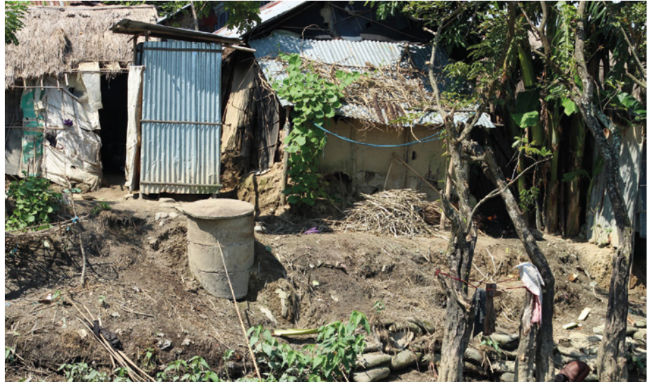
▶ Figure 16: Latrine installed on the slope of a rural household, left bare by erosion causing environmental and health risks (SanMarkS Project, Sunamganj, 2017, Md. Imran Nizami in IDE, 2022)
