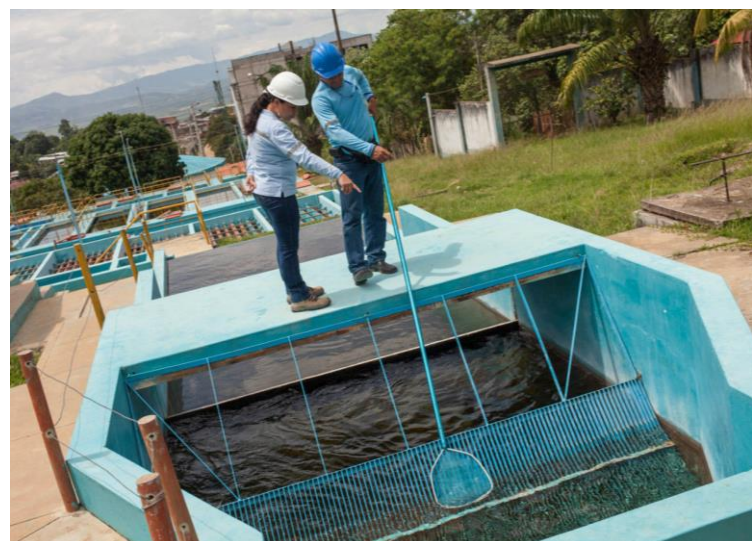
Drinking water treatment plants of the growing city of Tarapoto
