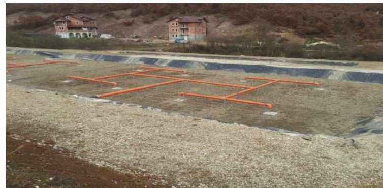
Construction of the Rural Waste Water Treatment Plant in Ternavc Village (spring 2013)
