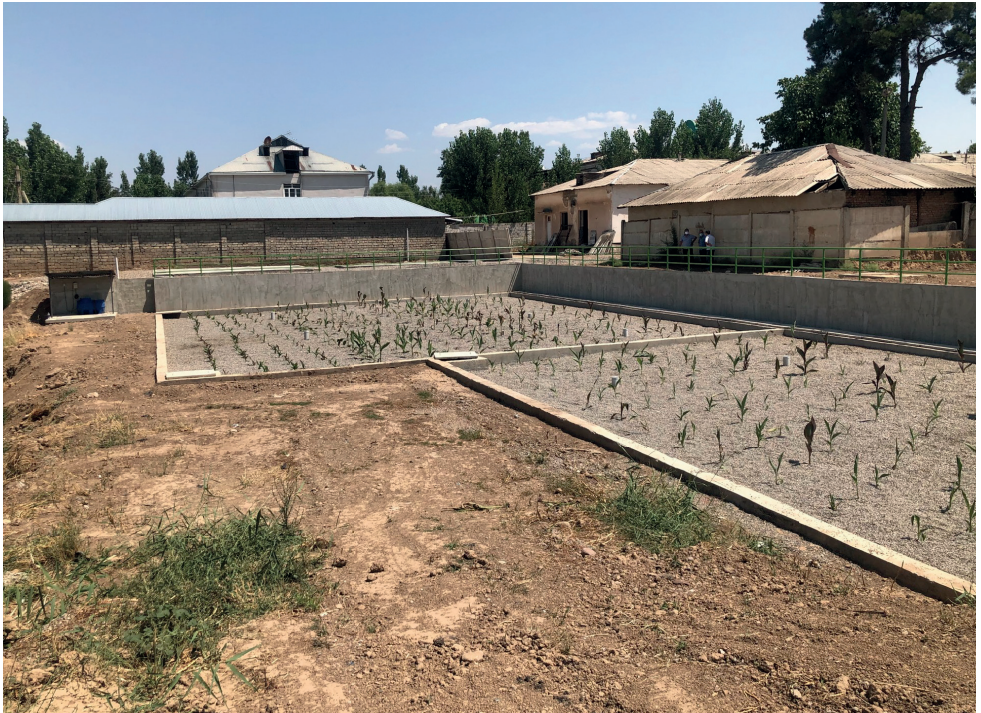
Planted gravel filter
