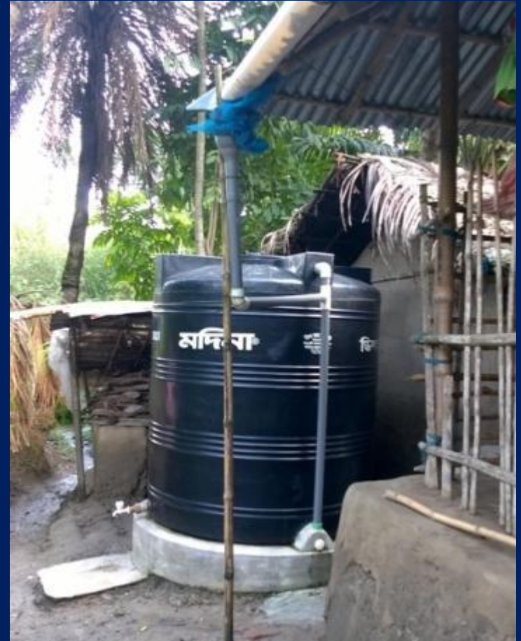
Rain Water Harvesting
