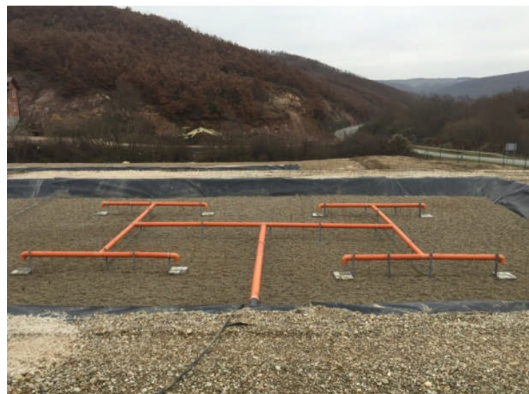
Wasterwater treatment plant in Kosovo
