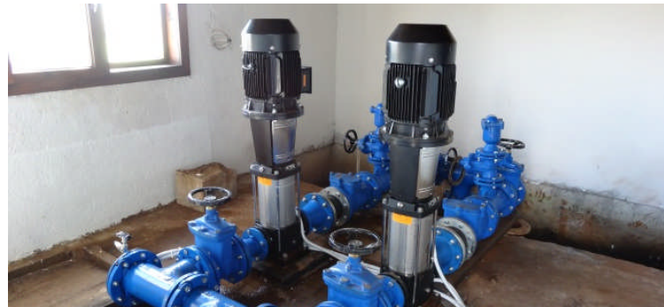
Rehabilitation of the pumping station of a well for drinking water in the municipality of Berovo
