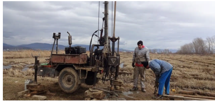
Drilling of boreholes for the geo-mechanical investigation on the construction site of the WWTP.
