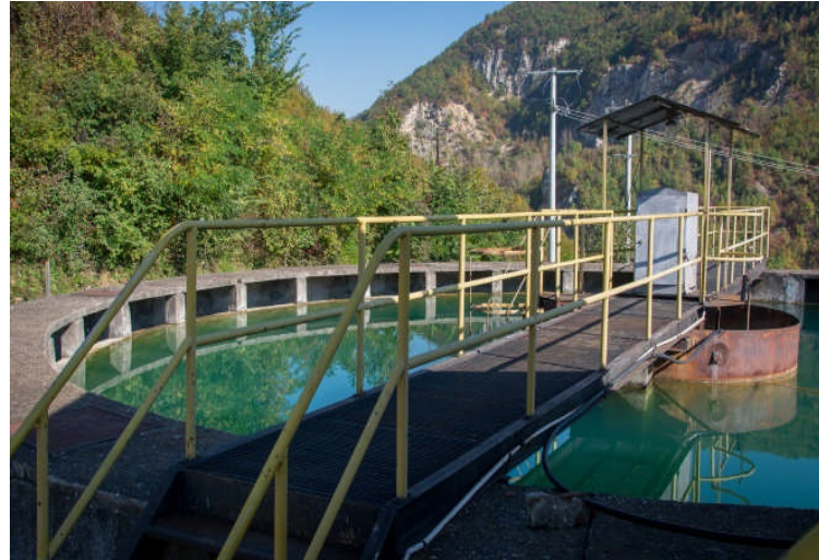
Drinking water treatment plant in Zenica
