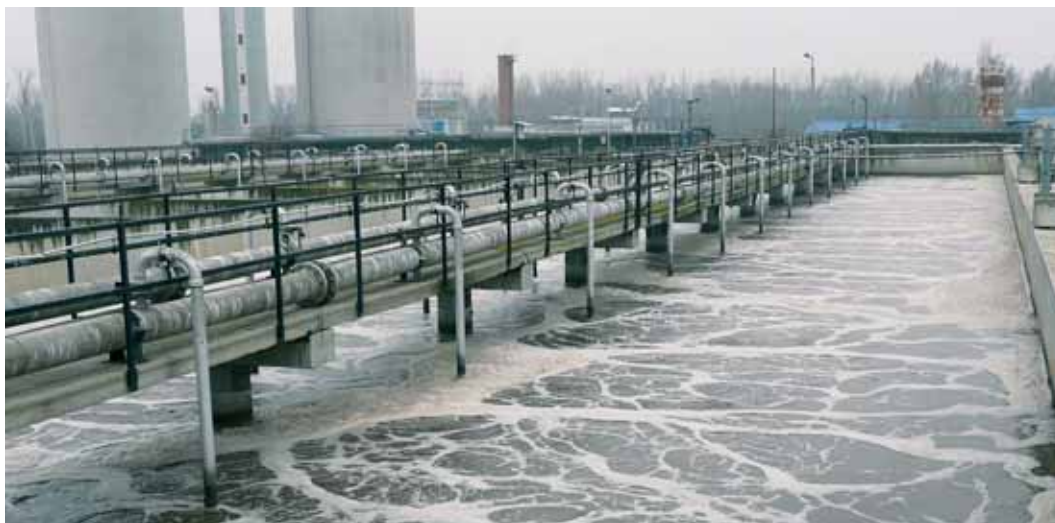
Sewage treatment plant in Debrecen, Hungary (Photo: SECO)
