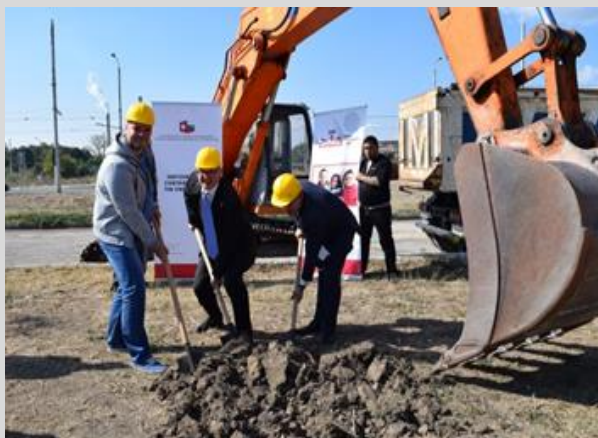
In September 2016, Sliven Municipality launched the construction of a childcare facility in the Roma neighbourhood Nadezhda. Apart from a nursery and kindergarten, the facility will host a Healthcare and a Culture Centres.
