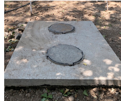
The urgency of the situation made DEWATS an ideal solution.
