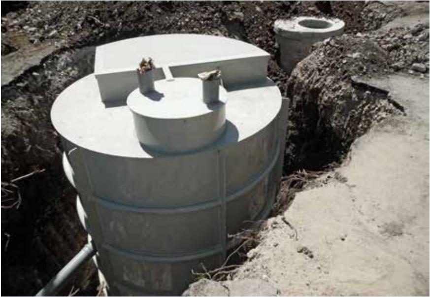
Example of school wastewater treatment in a package plant based on activated sludge
