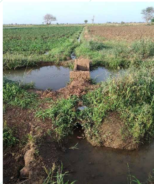
Figure 34: Broken distribution boxes and widened canal section at tertiary level
