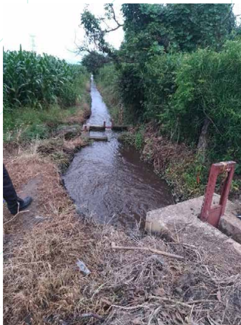
Figure 63: Flooded distribution box
