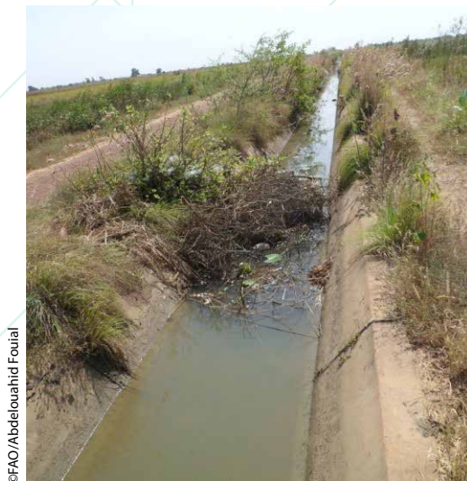
Figure 29: Vegetation breaking through the hairlines in the canal bed
