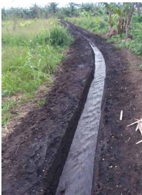
Figure 58: Lined quaternary canals with sufficient dimensions for water distribution
