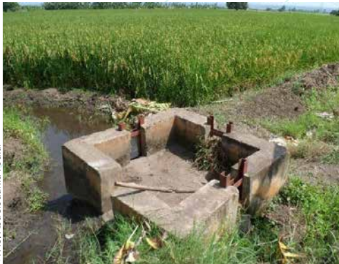
Figure 49: Destroyed distribution box, widened and unshaped quaternary canals
