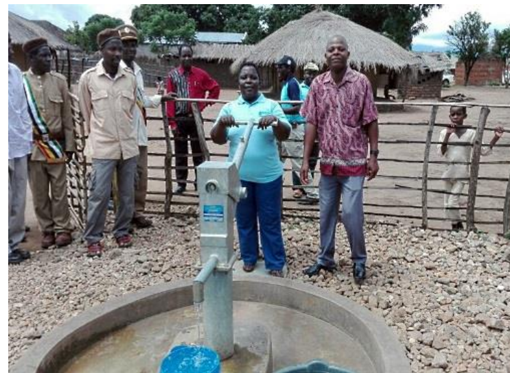
Water pumps funded by SA save lives and contribute to better health © SDC
